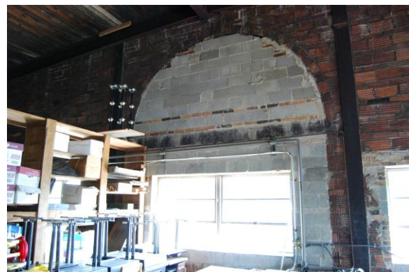
The openings of the domed windows were filled in with concrete blocks when Holy Trinity renovated the engine house.
