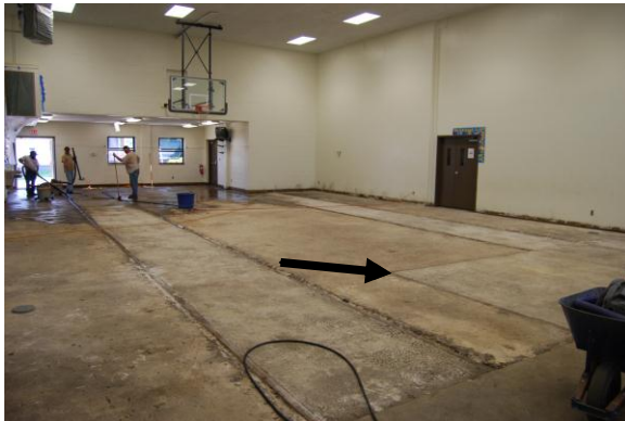
The railroad tracks and the outline of the pit used by LVRR mechanics to work underneath engines were visible after workers recently removed the flooring in Holy Trinity's social hall.
