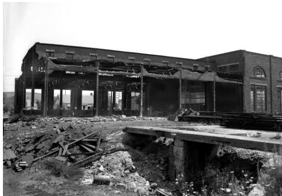
Two walls of the bay section of the engine house were removed at the beginning of the renovation project.
